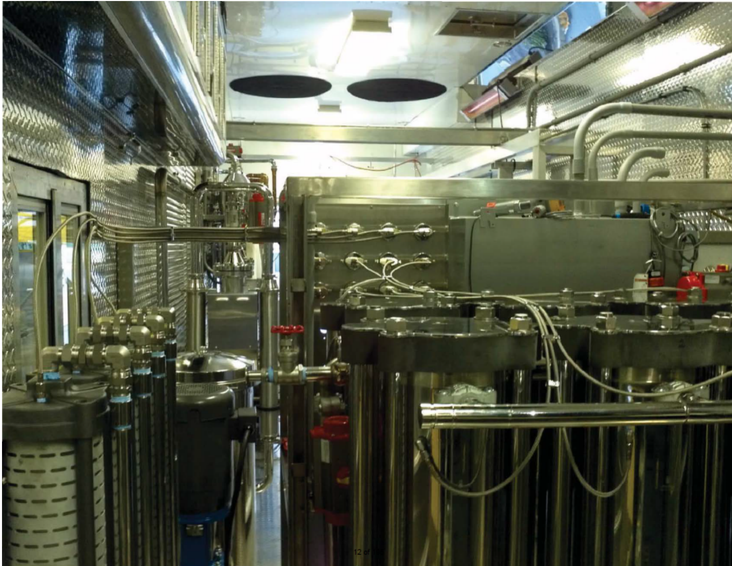
Inside water-power system
