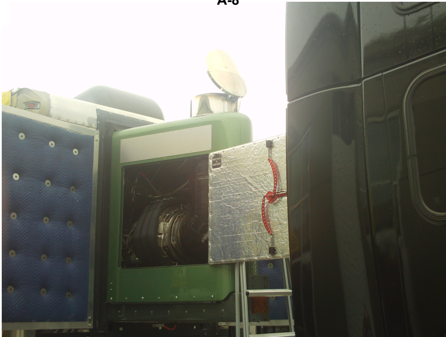
Syn-gas turbine and exhaust stack for expelling steam formed from syn-gas burn
