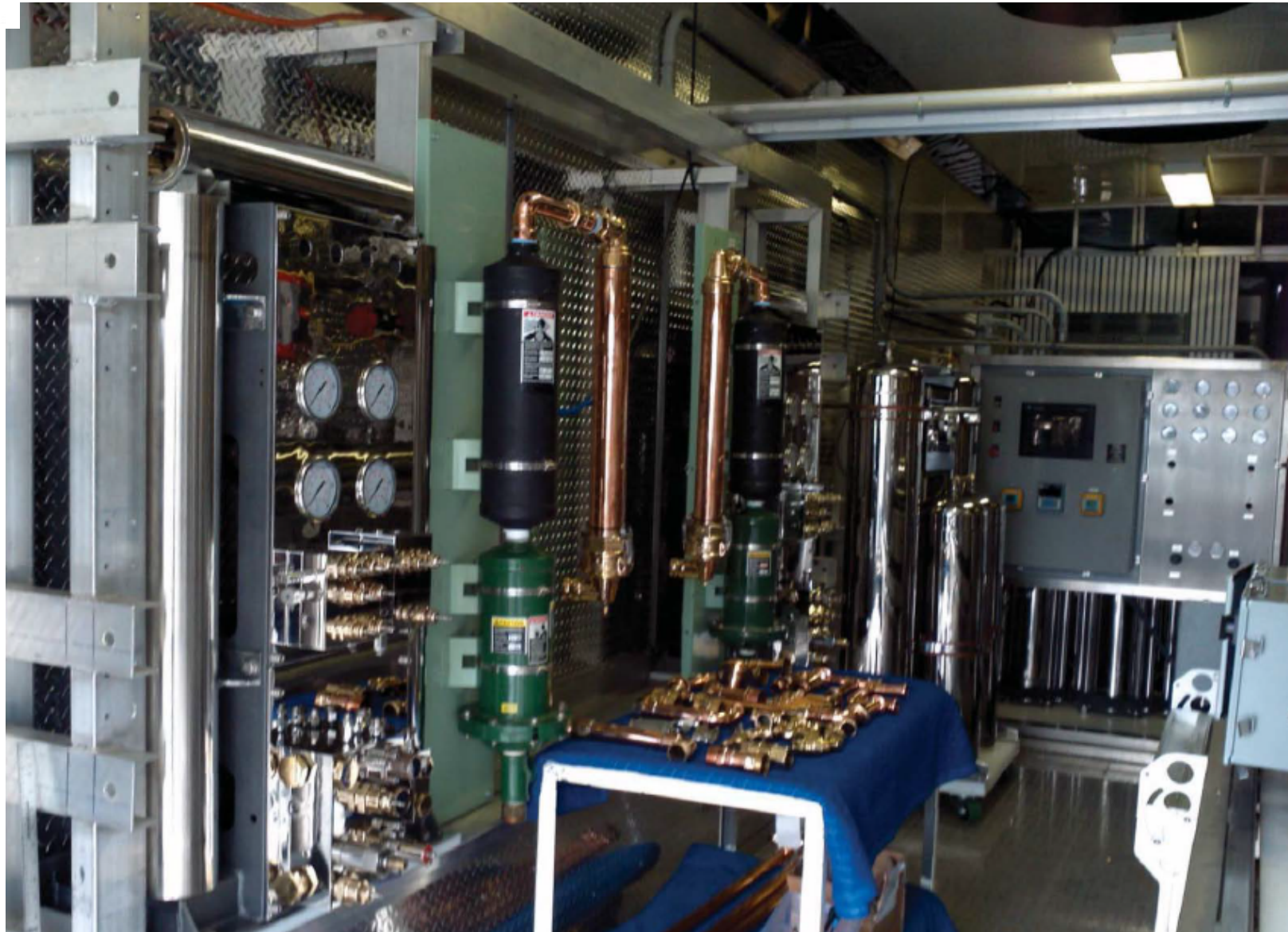
Inside water-power system
